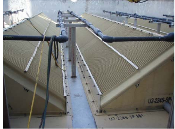
Figure 9.1-13 Typical Mist Eliminator System 27
